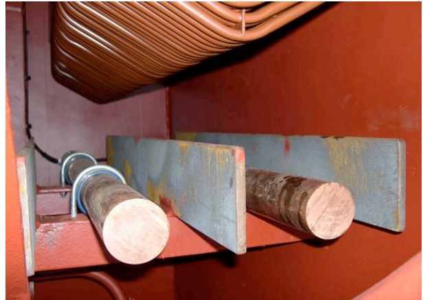
Figure 13. Copper rods (anodes) and steel (cathode) plates of the ICAF system mounted separately in the sea chest below the box cooler.
